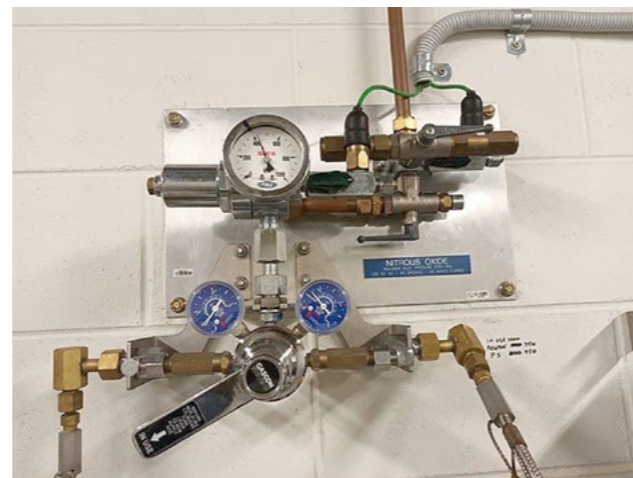
Figure 1: Main regulator at SCGH where original leak was found.
